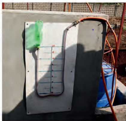
Manometer in Eigenbau
